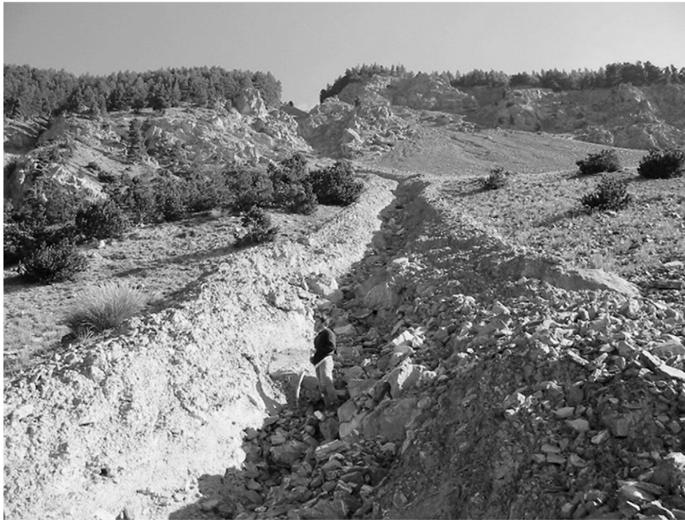
Fig. 6. Morphology of the eroded channel after the 2003 debris flow event at the Champerousse talus deposit in the upper part of the Faucon torrent.
