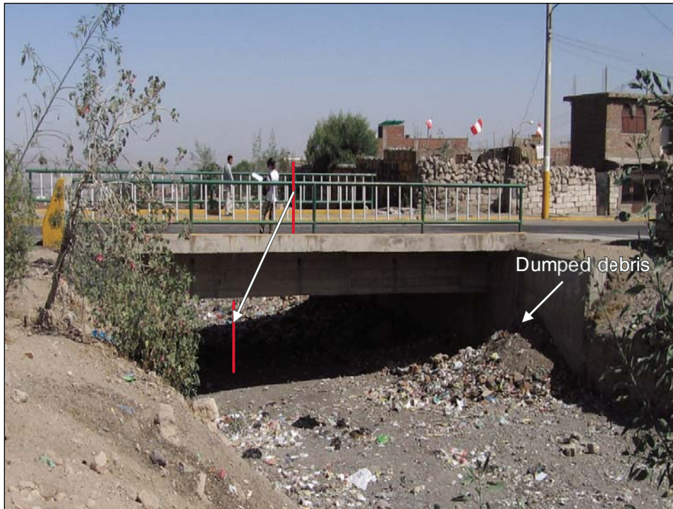
Figure 9. Huarangal pilot area: Infrastructure (roads and bridges). This bridge (Paucarpata–Mariano Melgar) along the Avenida Castilla is not only vulnerable to lahars because it is too low, but it could also increase hazard levels in surrounding areas by blocking the flow and creating overflow. Constant dumping of debris does not help either.
