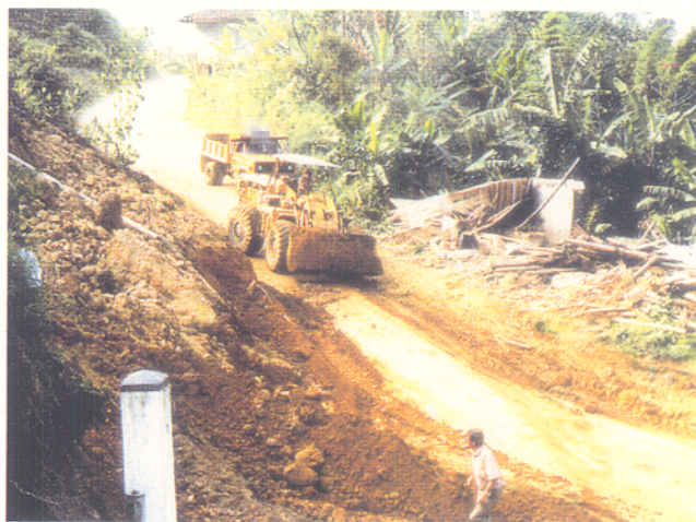
Figure 1. Example of landslide damage.
