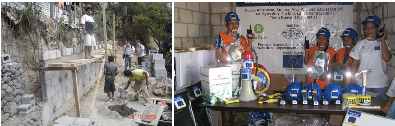
Figure: Support for community-based landslide risk reduction in RiskCity. Left: simple retaining walls are constructed by the local inhabitants with building materials supplied by the NGO. Right: equipment donated by the NGO for local landslide risk management: rain gauges, communication equipment etc.
