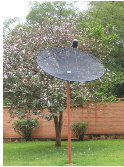
Satellite Dish installed at CGIS-NUR, Butare, Rwanda
